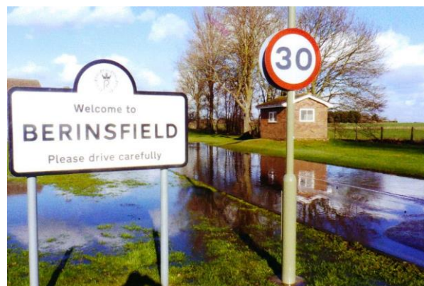
Recent ponding (2014) in lower Fane Drive was attributed to poorly-maintained drainage and ditches
