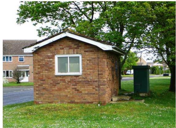
The sewage pumping station at the bottom of Fane Drive is stretched to capacity
